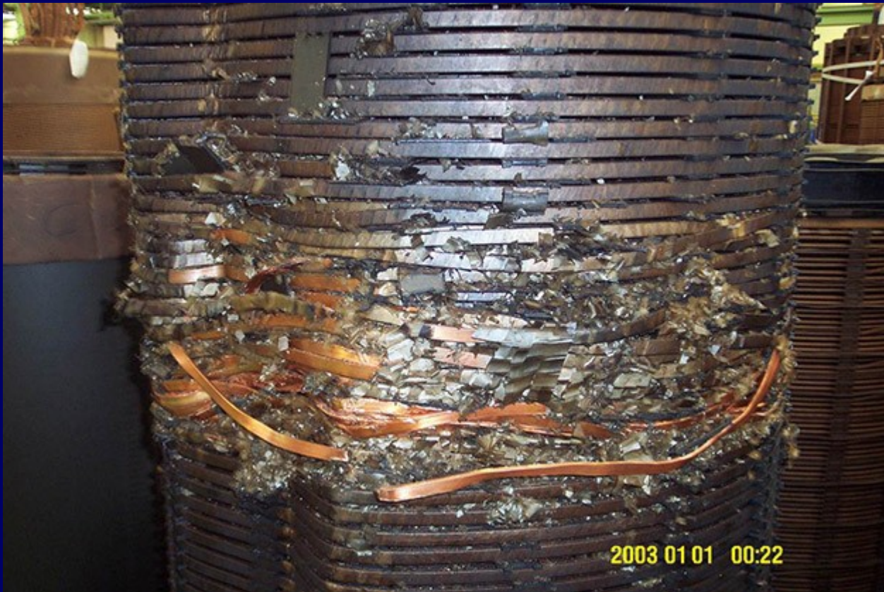
Power Transformer Winding Damage
